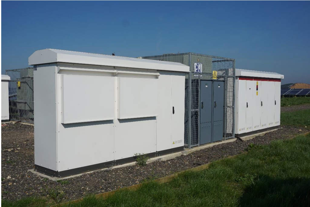
Plate 4 - Example of Solar Station located on a concrete pad surrounded by permeable hardstanding
